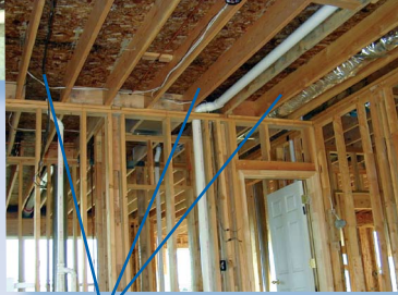
Holes between garage and house
