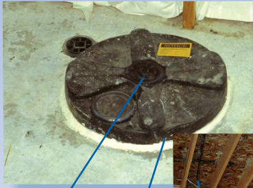
Open 3-inch hole No sealing at perimeter of cover
